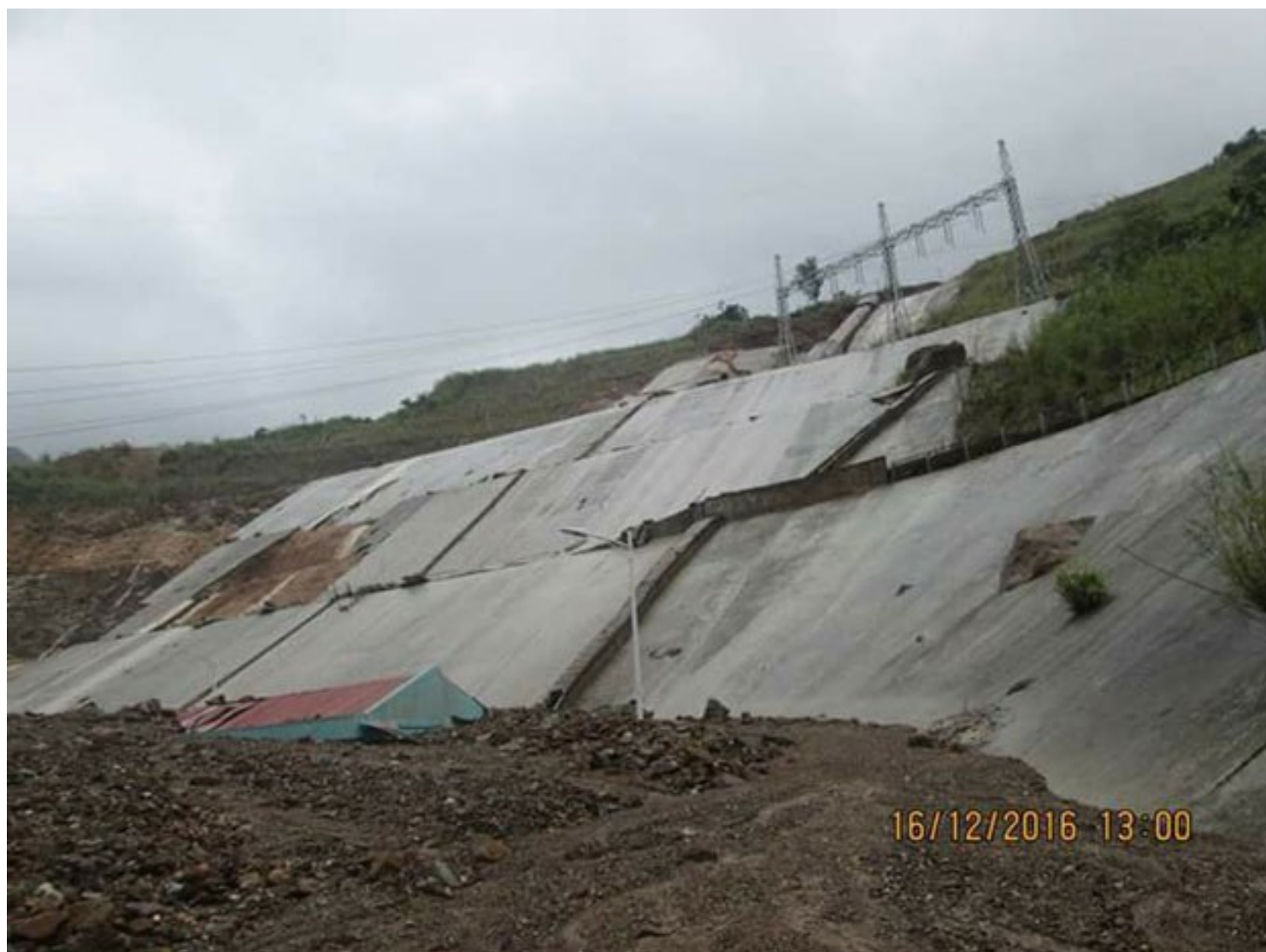
This image shows the Xekaman 3 dam after electrical production was shut down because of a break in the penstock.
